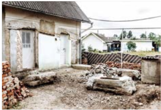
Many homes were damaged or destroyed.
